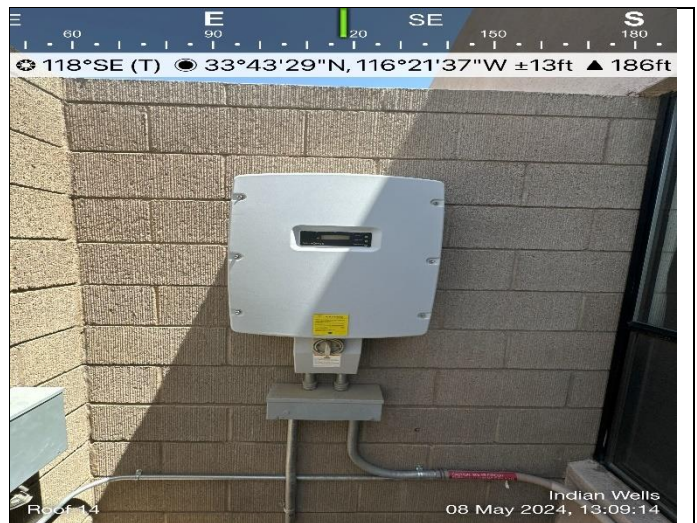
88. Roof 14 third inverter
