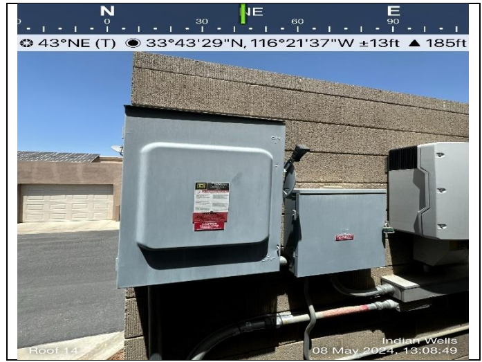
86. Roof 14 AC disconnect
