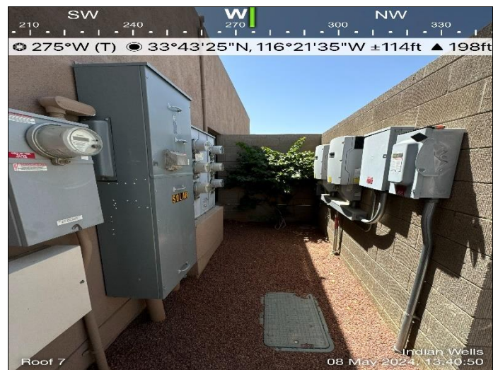
42. Roof 7 electrical corridor
