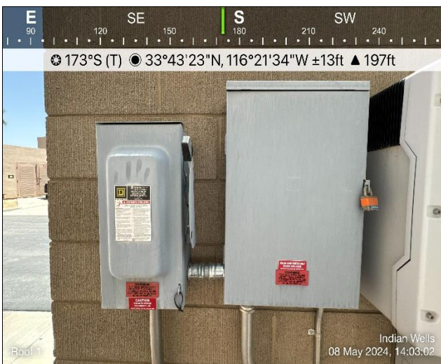
17. Roof 1 AC disconnect
