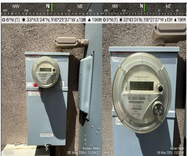
41. Roof 6 standalone meter
