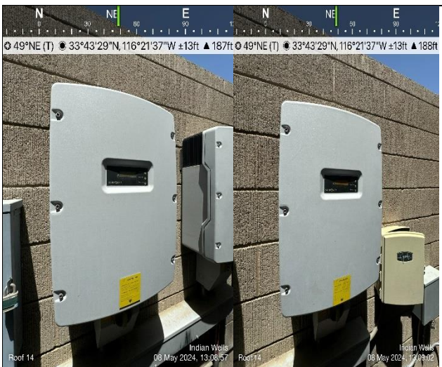
87. Roof 14 two inverters
