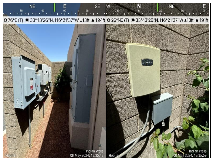
48. Roof 8 electrical corridor
