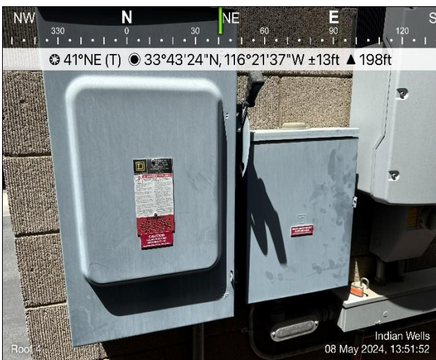
29. Roof 4 AC disconnect
