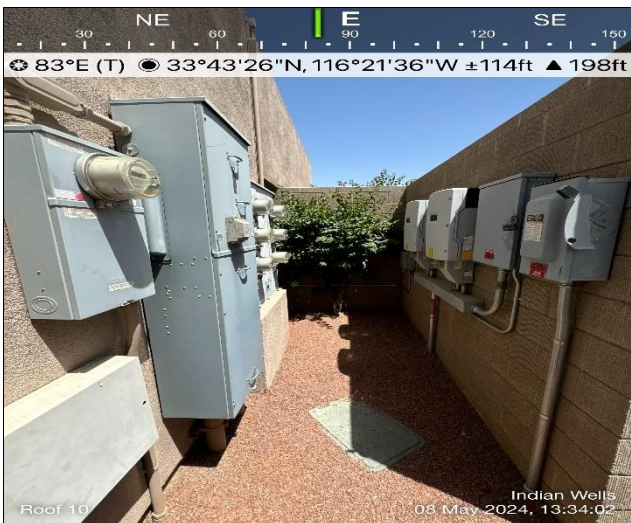
57. Roof 10 electrical corridor
