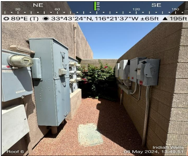
37. Roof 6 electrical corridor
