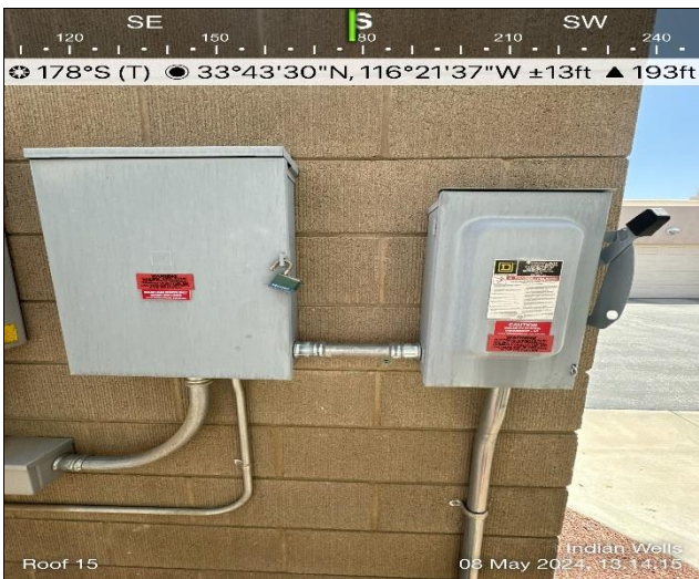
99. Roof 15 AC disconnect
