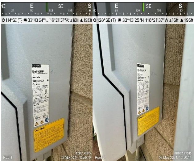
39. Roof 6 inverters label 7000W
