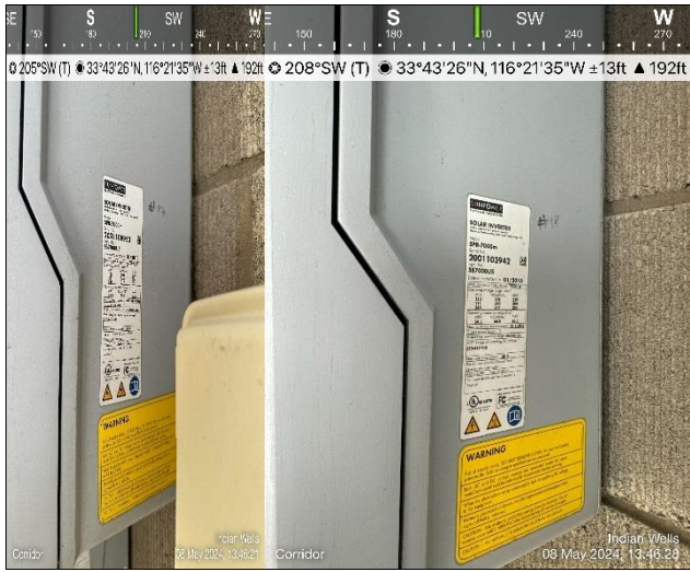
103. Corridor inverter label 7000W
