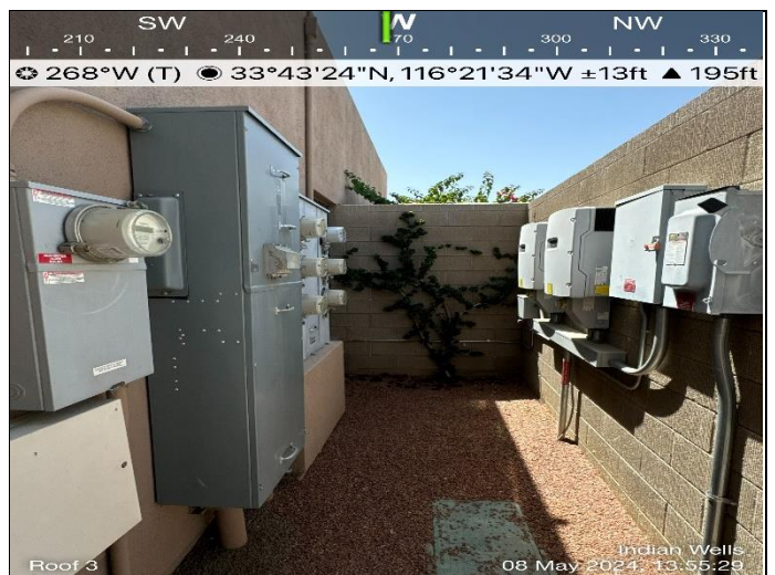
24. Roof 3 electrical corridor
