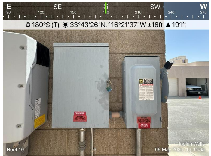
60. Roof 10 AC disconnect
