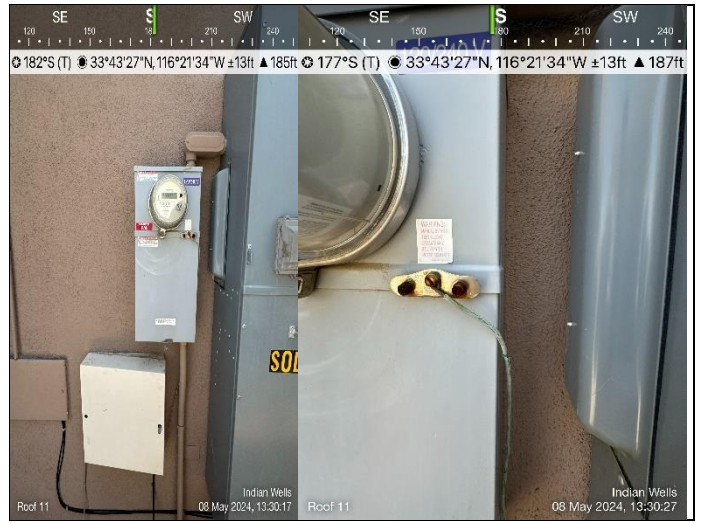
68. Roof 11 standalone meter
