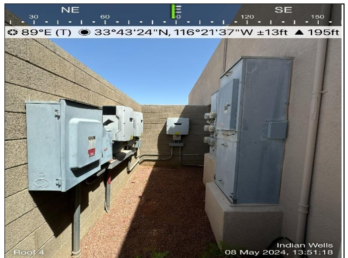
28. Roof 4 electrical corridor
