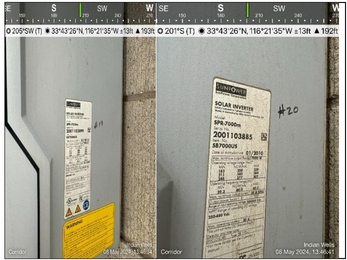
104. Corridor inverter label 7000W
