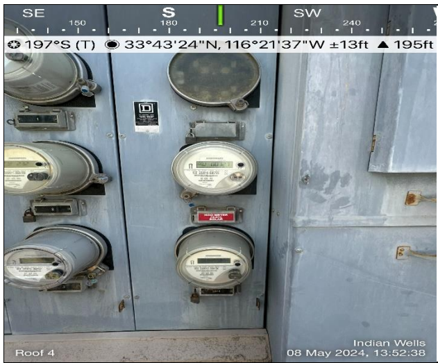
31. Roof 4 generation meter
