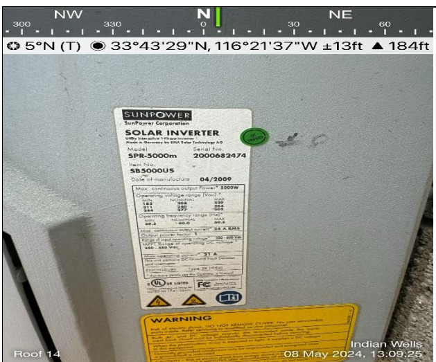
89. Roof 14 inverter label 5000W
