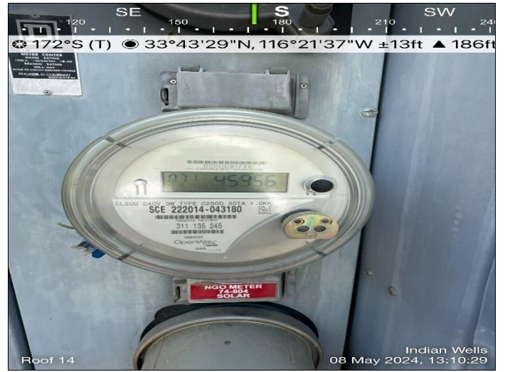
92. Roof 14 generation meter
