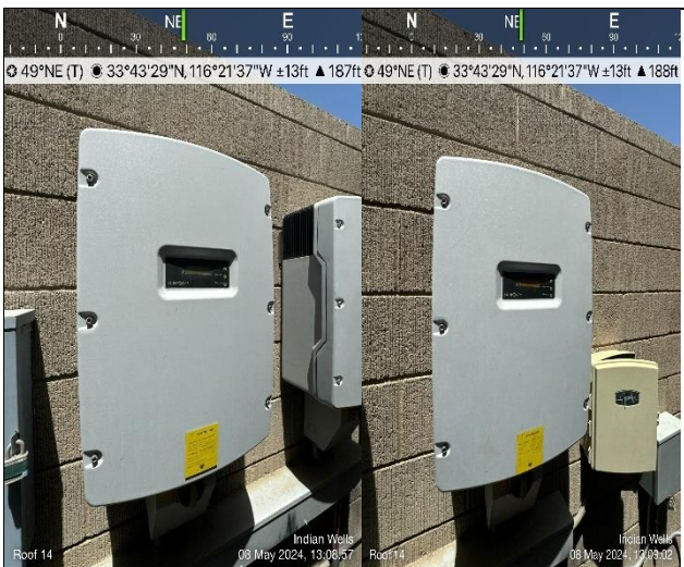
87. Roof 14 two inverters
