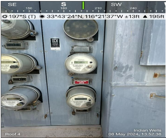
31. Roof 4 generation meter
