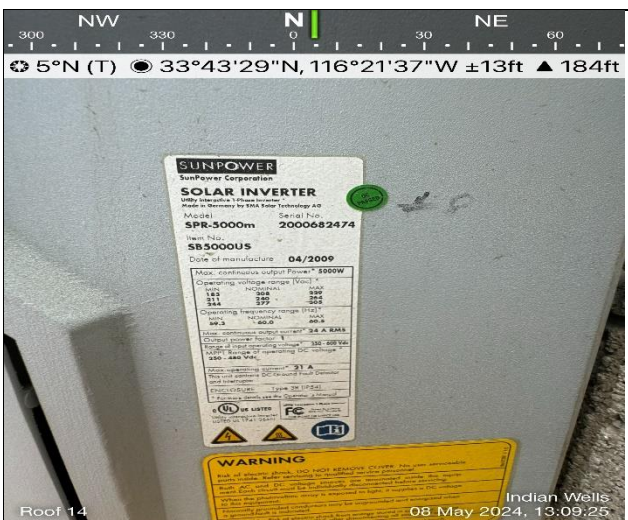
89. Roof 14 inverter label 5000W
