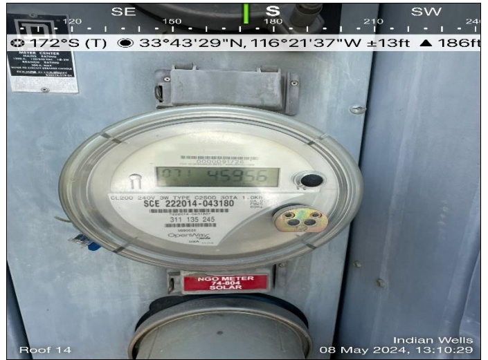
92. Roof 14 generation meter
