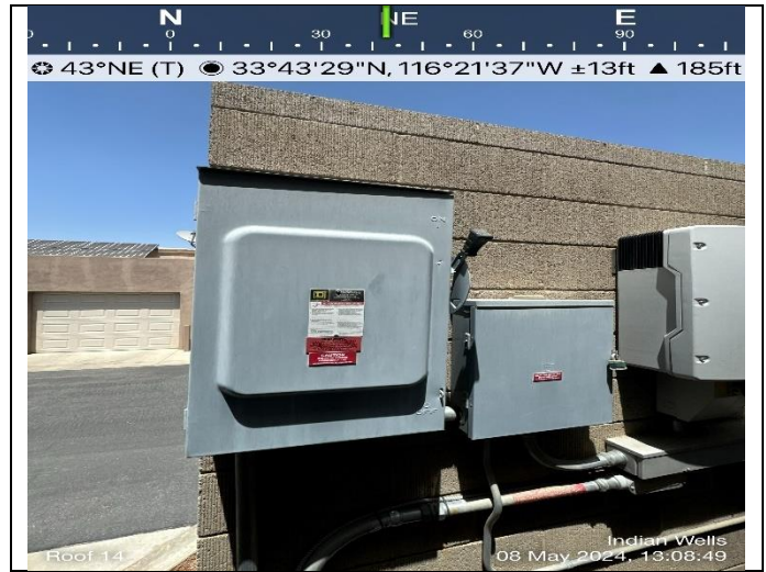
86. Roof 14 AC disconnect
