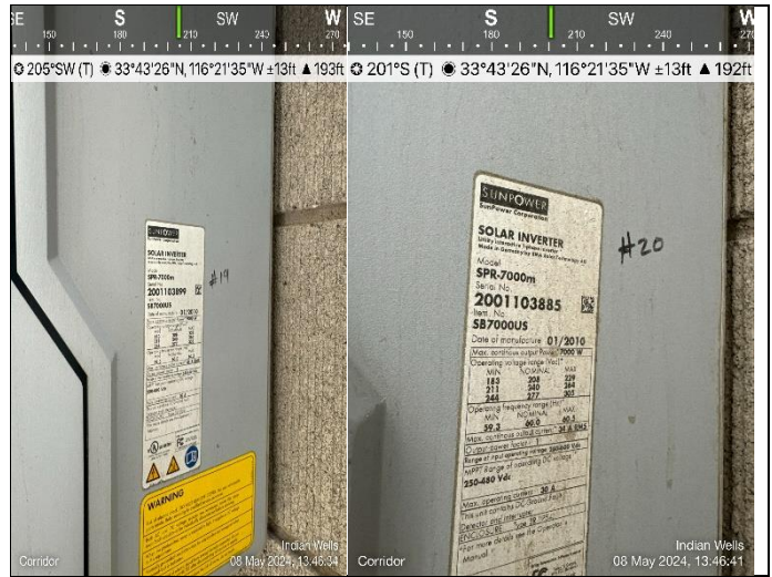
104. Corridor inverter label 7000W
