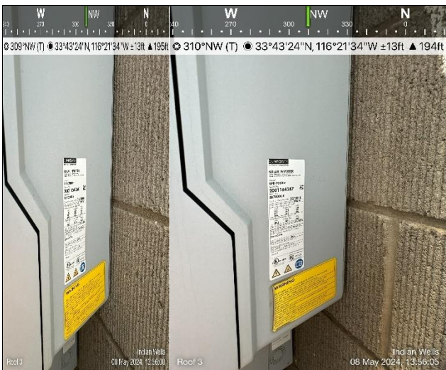
27. Roof 3 inverters label 7000W
