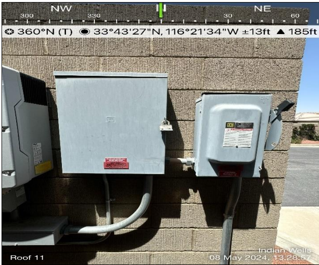
67. Roof 11 AC disconnect
