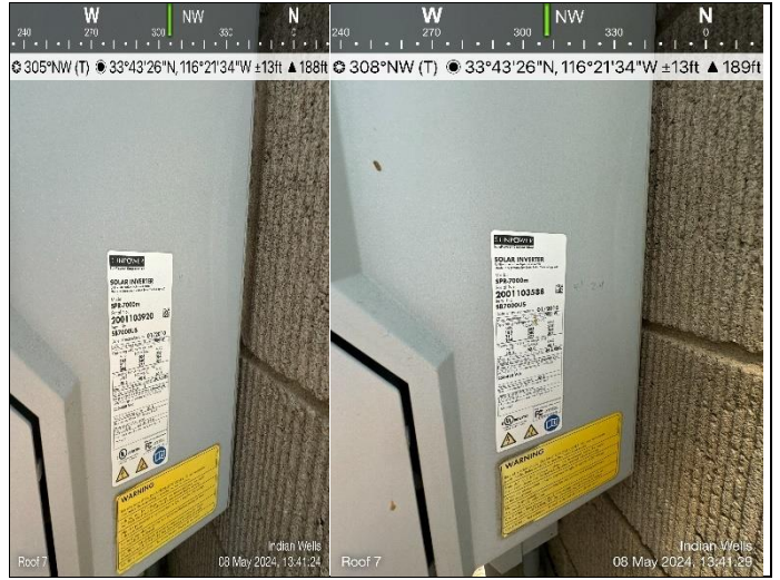
44. Roof 7 inverters label 7000W
