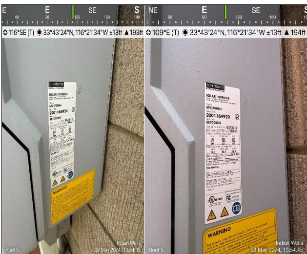
35. Roof 5 inverters label 7000W
