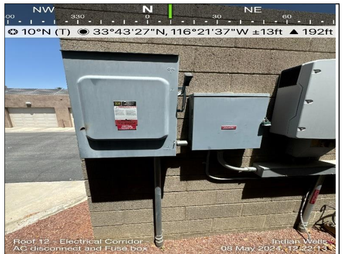
70. Roof 12 AC disconnect
